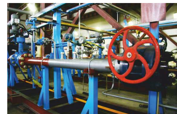
2010 - Block of inlet lines at Yarakinskoye oil and gas field OOO Irkutsk Oil Company. Part of process pad
