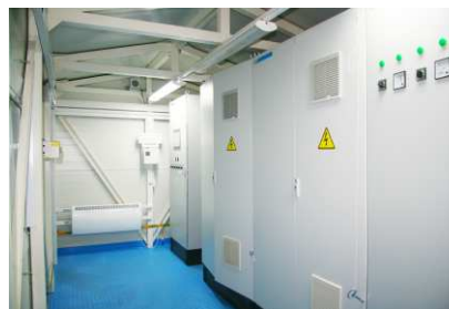
2009 - Prefabricated building for control room of MPS at Katangli oilfield OOO RN-Sakhalinmorneftegas, OAO NK Rosneft. Inside view
