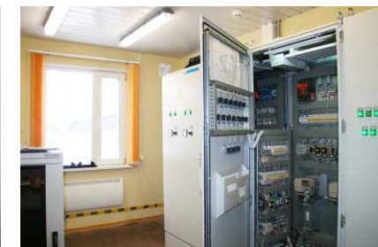
2010 - Administrative and on-site quarters for Crude Oil Acceptance and Delivery Station of Oil Refinery in the village of Semiluzhki, Tomsk Oblast, OOO Tomskneftepererabotka. MCC room
