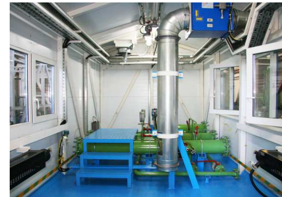
2010 - UUV of Talinskoye pad of Krasnoleninskoye oil and gas field, OAO TNK-Nyagan, OAO TNK BP. View from main entrance
