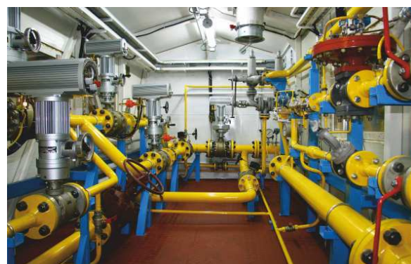
2010 - Gas reduction unit at Boatasino pad of OOO RN-Sakhalinmorneftegas, NK Rosneft. General View
