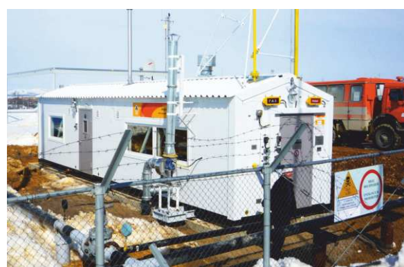
2010 - Gas reduction unit at Boatasino pad of OOO RN-Sakhalinmorneftegas, NK Rosneft. Installation of products at site
