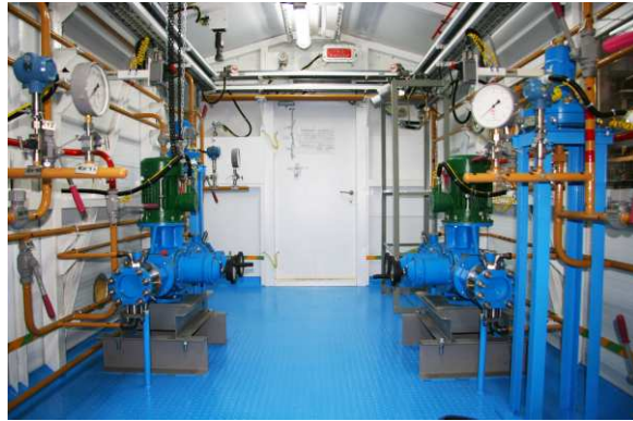
2010 - BPS for liquified petroleum gas of Kazanskoye oil and gas field OAO Vostokgasprom, OAO Gazprom. General View
