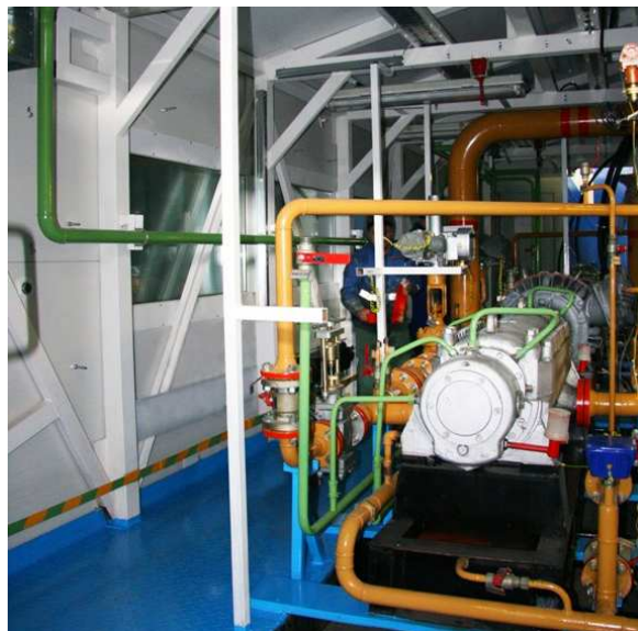
2009 - BPS for oil pumping at Katangli of OOO RN-Sakhalinmorneftegas, NK Rosneft. Pump
