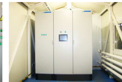
2010 - Control room for Gas reduction unit at Boatasino pad, OOO RN-Sakhalinmorneftegas, NK Rosneft. Inside view
