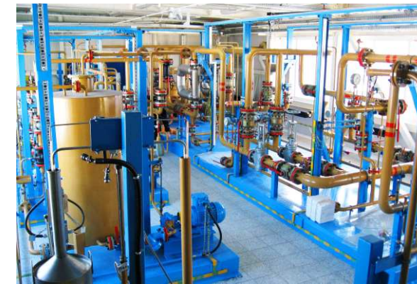
2010 - SIKN for Crude Oil Acceptance and Delivery Station of Oil Refinery in the village of Semiluzhki, Tomsk Oblast, OOO Tomskneftepererabotka. General View
