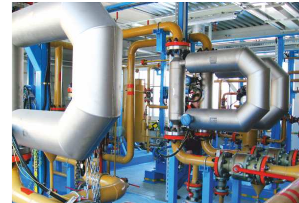
2010 - SIKN for Crude Oil Acceptance and Delivery Station of Oil Refinery in the village of Semiluzhki, Tomsk Oblast, OOO Tomskneftepererabotka. Block of Metering Lines
