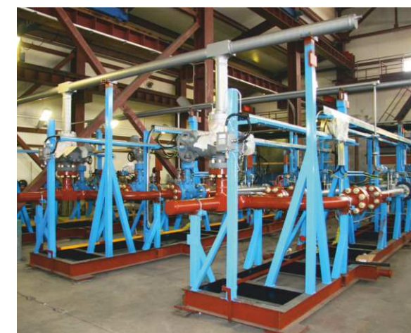
2010 - Block of inlet lines at Yarakinskoye oil and gas field OOO Irkutsk Oil Company. General View
